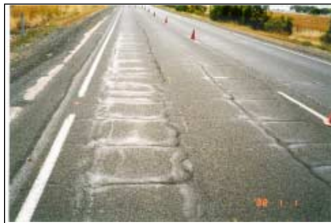
Figure 4 – Failed cement stabilised pavement (4% Cement), SA
