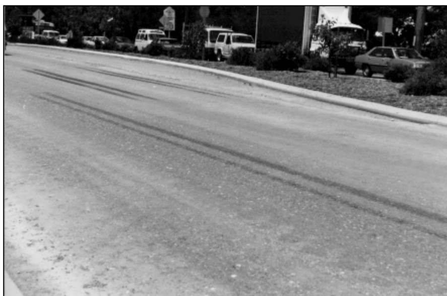
Figure 6 – Skid marks on stabilised surface of Nicholson Rd
