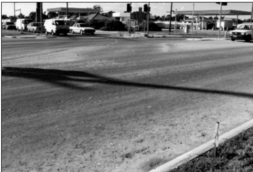
Figure 5 A view of the surface before sealing at the intersection of Nicholson and Spencer Roads.
