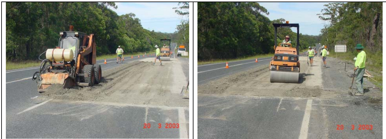
Figure 3 View of skidsteer and smooth drum roller system for small pavement patch repairs.
