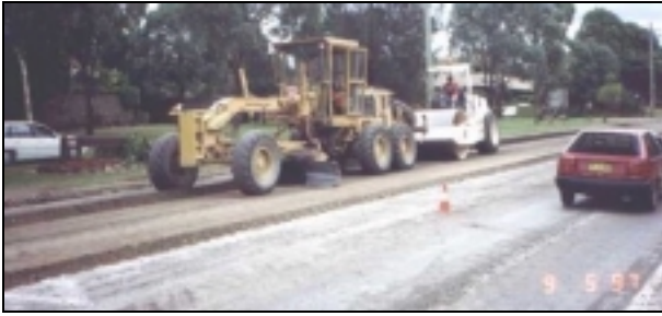
Figure 10 Full-width stabilisation in one day with one lane open to traffic (Avoca Road).
