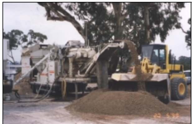
Figure 2 Foamed bitumen stabilisation using a mobile batch plant. The material is placed using conventional road making and/or asphalt laying equipment.
