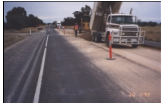
Figure 8 Plant-mix foamed bitumen stabilised material being layed using conventional road making equipment.
