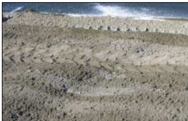
Figure 8 Single pass mixing is likely to lead to streaks of binder in the pulverised material.
