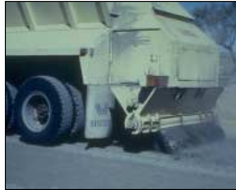
Figure 5 The binder being spread in front of the reclaimer before first stage mixing.
