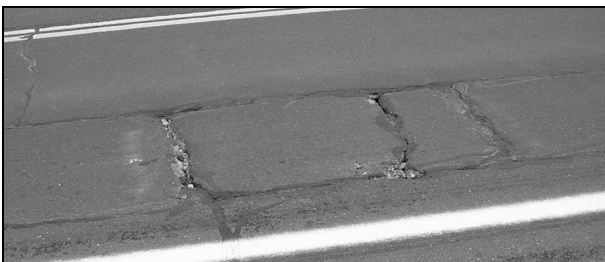
Figure 1 Stabilised pavement showing block cracking due to weak subgrade region.
