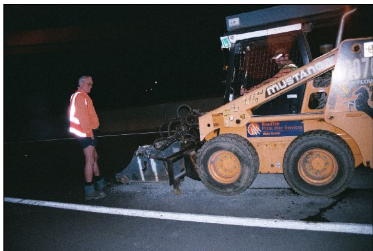
Figure 1: The use of the profiler attachment to a skidsteer can provide a breakdown of the material during site investigations.
