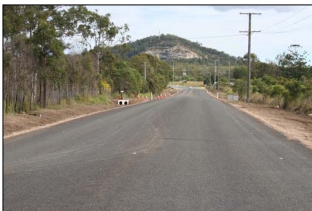
This foamed bitumen stabilised road was inundated for several days after the July floods..
