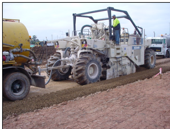
The stabiliser mixing quicklime into the thick clay subgrade followed by the addition of water to optimise the subgrade.
