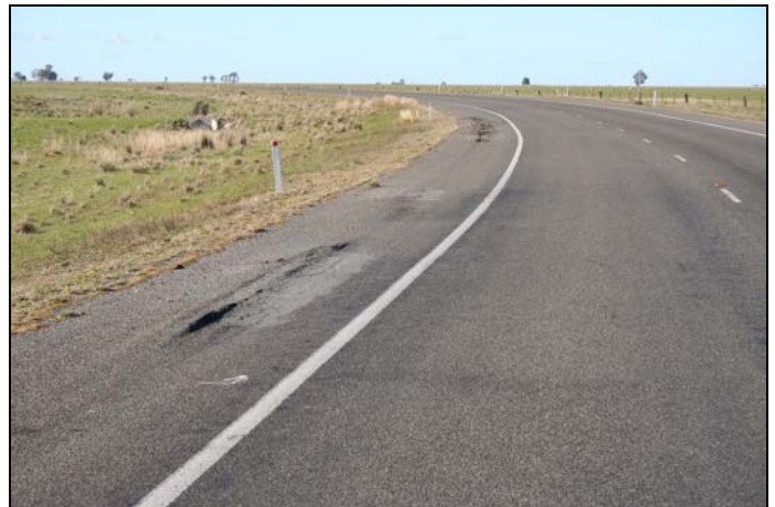
The shoulder material has become weak after rain & yet the stabilised carriageway is still functioning without any distress.
