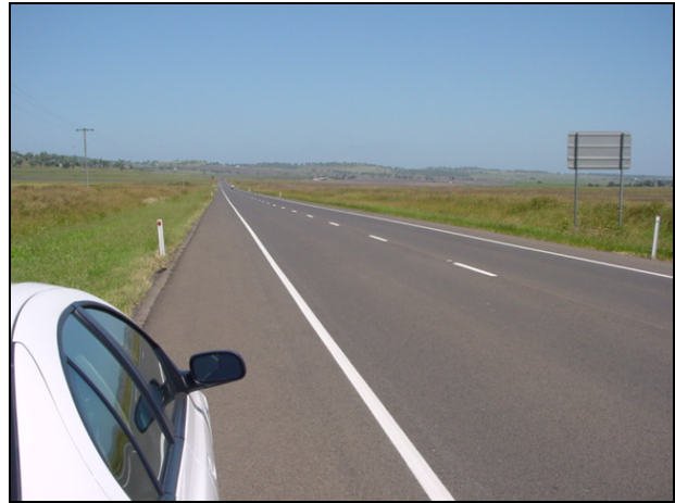
This section of the Cunningham Highway has the black soil subgrade stabilised with lime.
