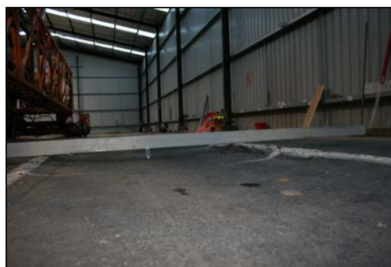
View of deflected cement material pavement after about 700,000 ALF cycles.
