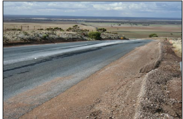
Foamed bitumen stabilisation used for rehabilitation of the Sturt Highway at Accommodation Hill (SA).
