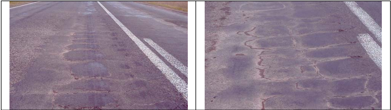
Figure 3 A view failed stabilisation patching on the Hamilton Highway at Derrinallum. (Photo taken in May 2003)
