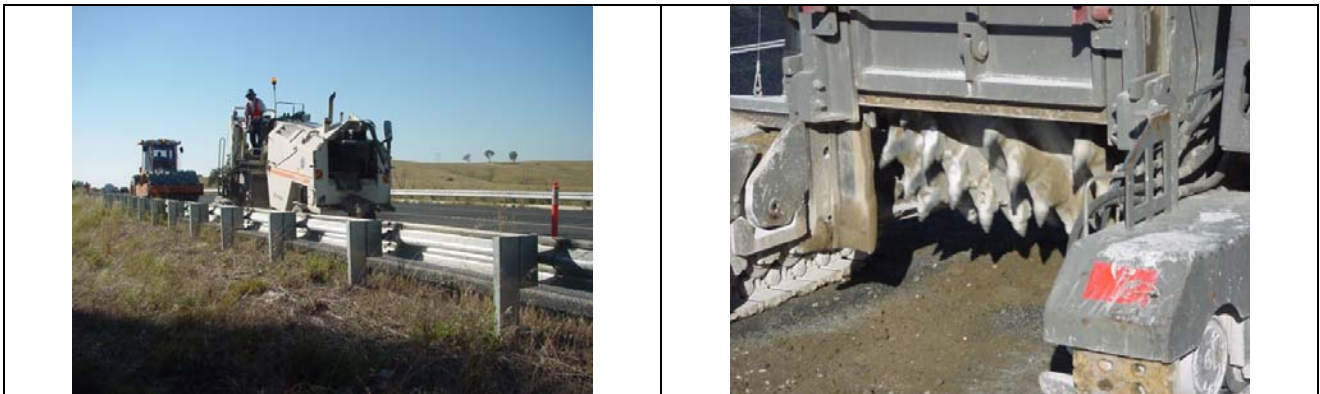
Figure 2 A profiler incorrectly used for road stabilisation in NSW due to the poor mixing quality. (Photo taken in March 2000)
