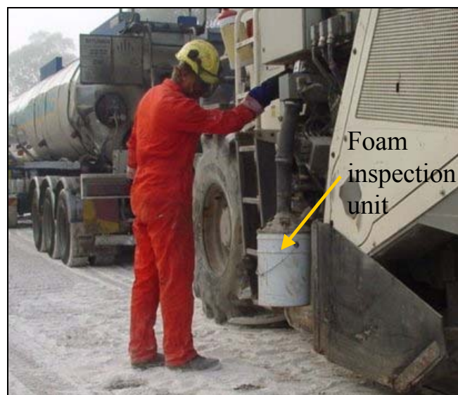
Figure 8 Operator assessing foaming nozzle operation from special inspection system on the reclaimer.
