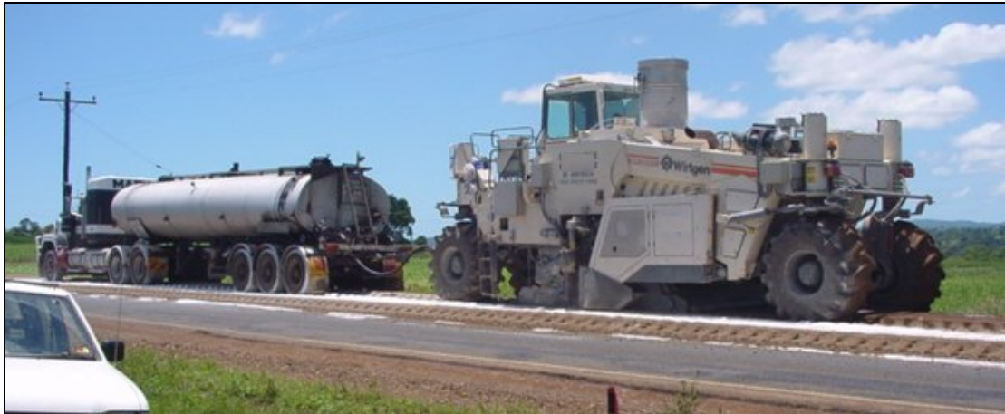
Figure 7 The Wirtgen WR2500 reclaimer coupled with a bitumen tanker providing hot bitumen to the reclaimer.
