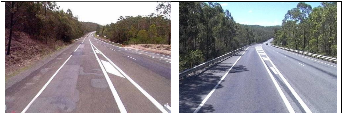
Figure 1 Insitu foamed bitumen stabilisation trial at Cooperabung, NSW prior to stabilisation (LHS) and the road after construction in January 2004 (RHS).
