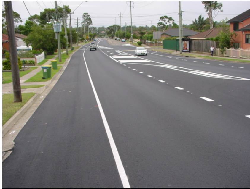
Figure 2 Foamed bitumen carried out in the trafficable lanes of Fitzwilliam Street, Toongabbie with a new asphalt surface from kerb to kerb.
