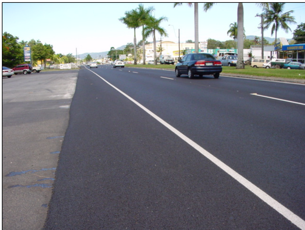
Figure 1 Water draining on the kerbside of an SMA layer on a foamed bitumen base.
