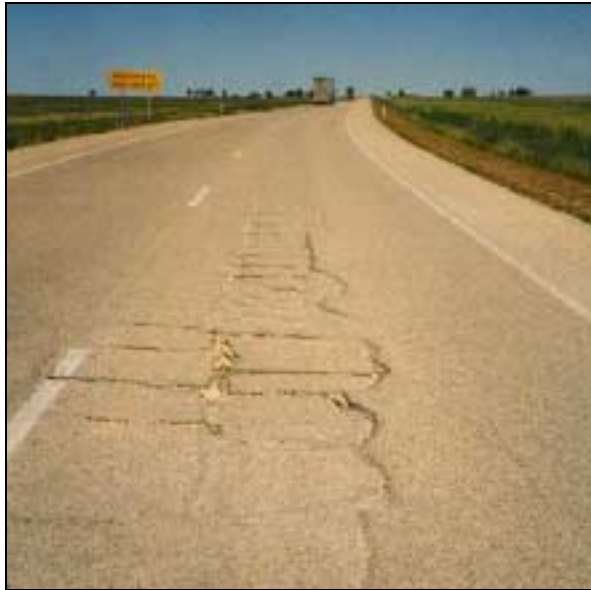
Figure 5 Very stiff and thin stabilised pavements are likely to crack when built on wet and weak subgrades. (Photo courtesy of RTA)
