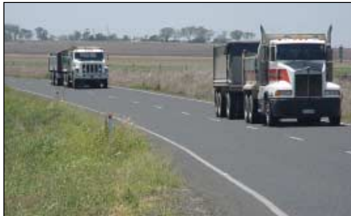
Figure 3 With the shoulder unsealed, water is allowed to pond in the outside wheel path and this increases pavement damage.
