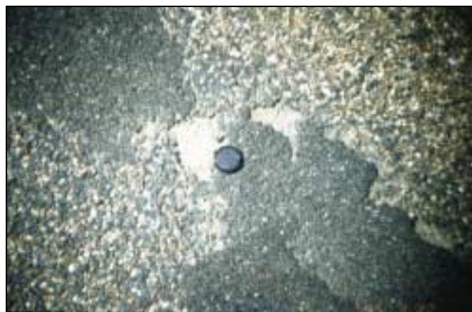
Figure 4 Bitumen seal “blow-out” as a result of salt under the seal. (Photo courtesy of RTA)
