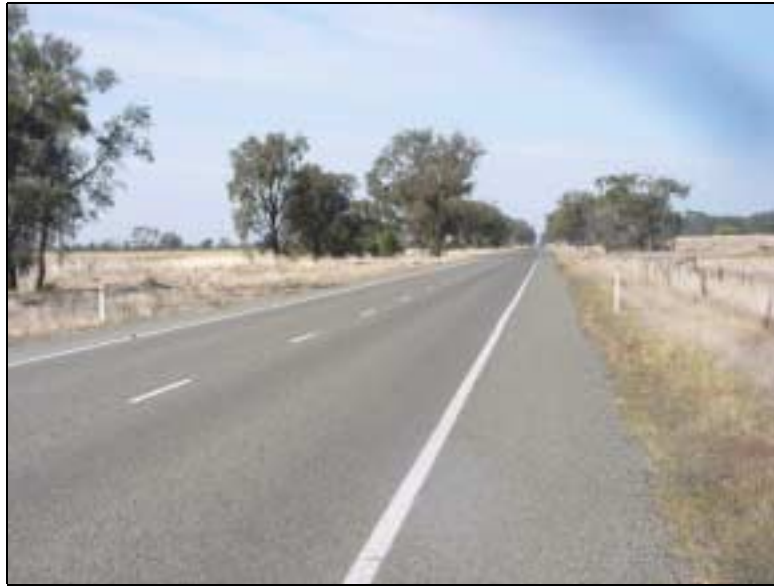
Figure 11 A section of the Riverina Highway where the upper 200 mm of the road base has been stabilised with Polyroad.
