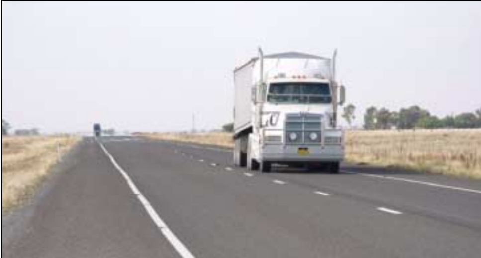
Figure 2 The seal now extends well past the lane markings to increase safety and reduce the ingress of water into the pavement material. Newell Highway, just north of Jerilderie (NSW).
