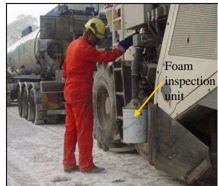
Figure 3. Operator assessing foaming nozzle operation from special inspection system on the reclaimer.
