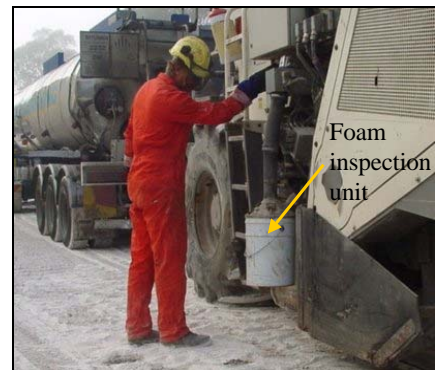
Figure 3. Operator assessing foaming nozzle operation from special inspection system on the reclaimer.
