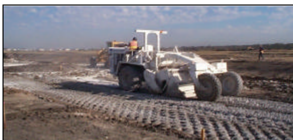
Figure 1 Lime stabilisation of a weak subgrade for a light trafficked street in a new subdivision.
